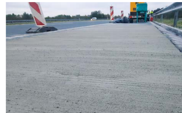
Renovation of shoulder with MORTAR MIX on a busy transit route in Poland
